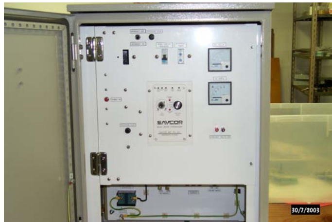
Savcor Products supplies a wide range of transformer rectifiers custom built to suit customer requirements
